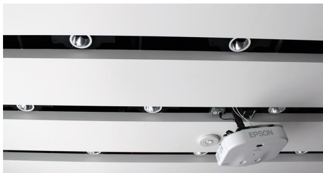
Figure 3: Recessed ceiling lights. Lights such as these are traditionally difficult to meter due to limited access to their wiring and uncertainty about the topology of the lighting circuit. Our Gecko sensors are easily and unobtrusively installed in fixtures such as these. See Figure 2(c) for a closeup view of the sensor mounting.
